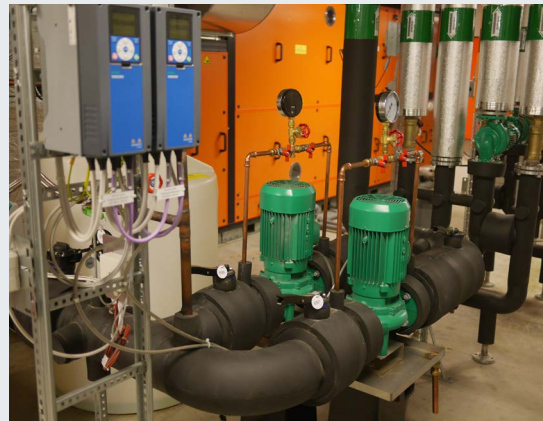
Fig. 2: One issue identified in the Studenthuset GSHP system was excess pumping power. Photo credit: J.D. Spittler
